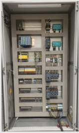
CE-Label Electrical System
