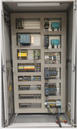
CE-Label Electrical System
