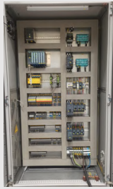
CE-Label Electrical System
