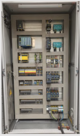
CE-Label Electrical System
