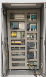
CE-Label Electrical System
